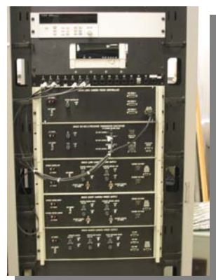
RACK 2 FRONT PANELS
